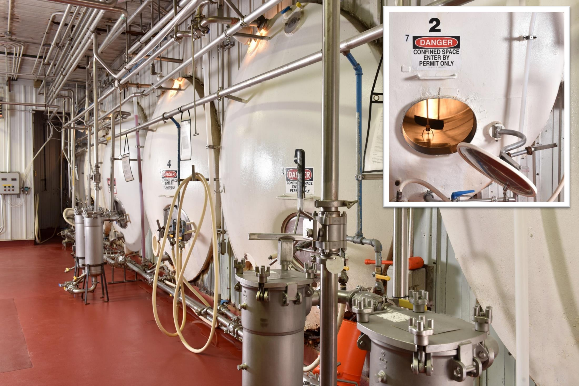
Liquid plasma is stored on site in insulated, stainless steel tanks.
